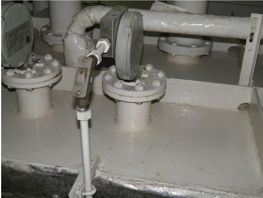
Figure 4: The mechanism of the level gauge on top of No 2 Waste Oil Settling tank.
