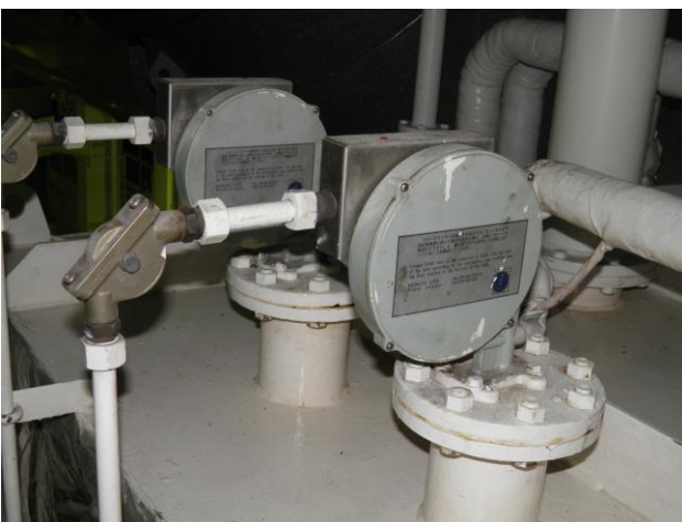
Figure 8: The device for the wire scale reduction fitted on top of the tank.
