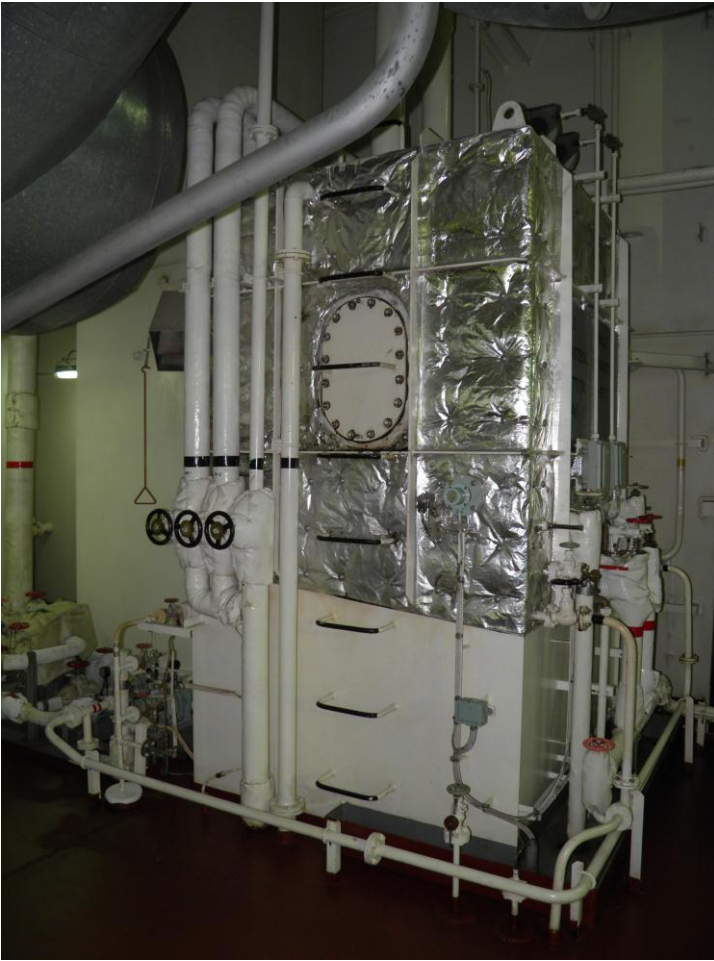
Figure 7: The manhole of No 1 W.O.S. Tank fitted at the fore side of the tank.
