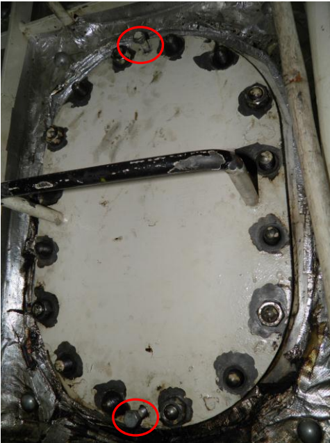
Figure 10: The manhole cover of No 2 Waste Oil Settling Tank and the two jackscrews fitted on the top and bottom side.
